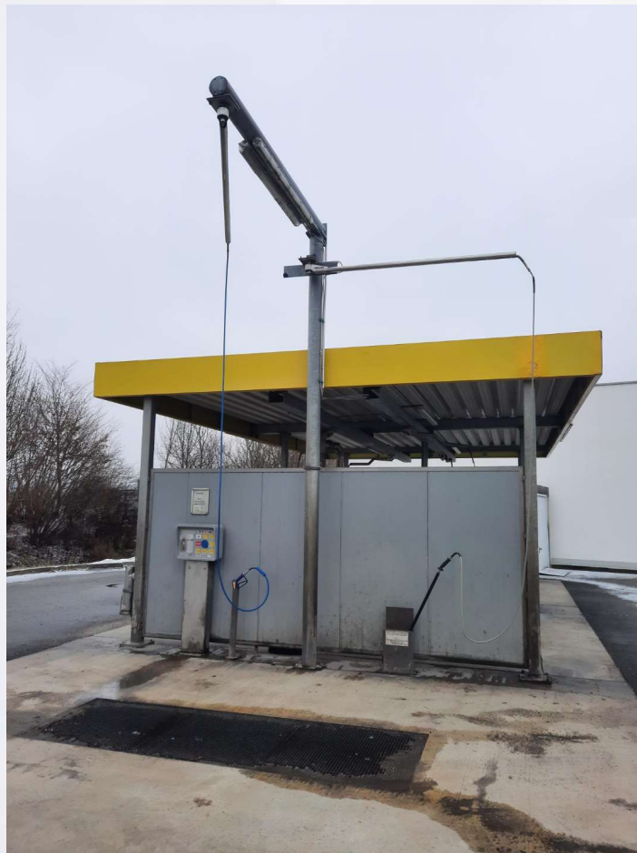
Altanlage / Existing Installation
